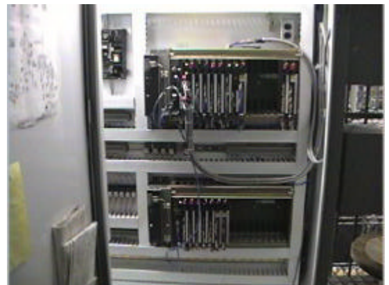
Figure 4 - PLC Control Panel
