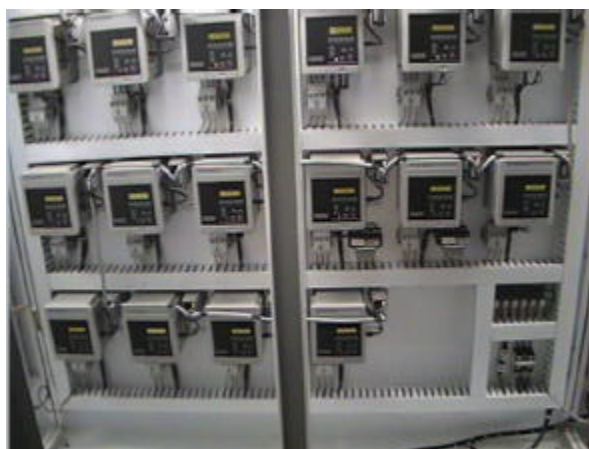
Figure 5 - Large VFD Drive Panel
